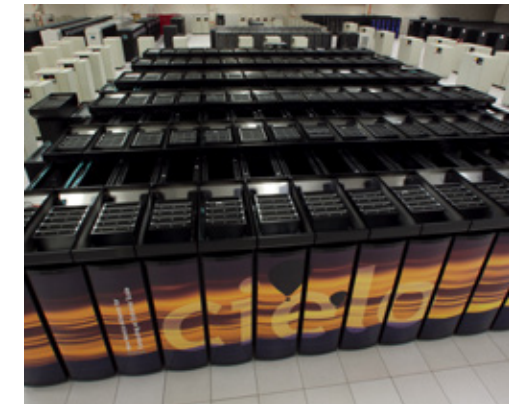
New Mexico ACES Cielo Platform 2011-2016.
