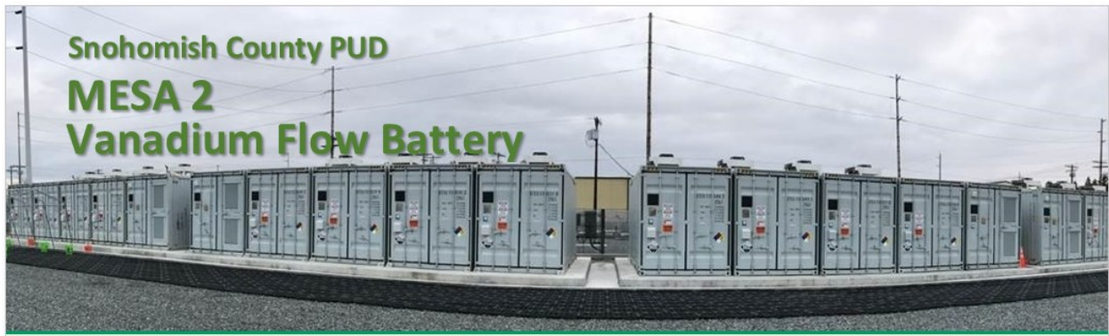
Figure 2. MESA 2 2-MW, 8-MWh FBESS
