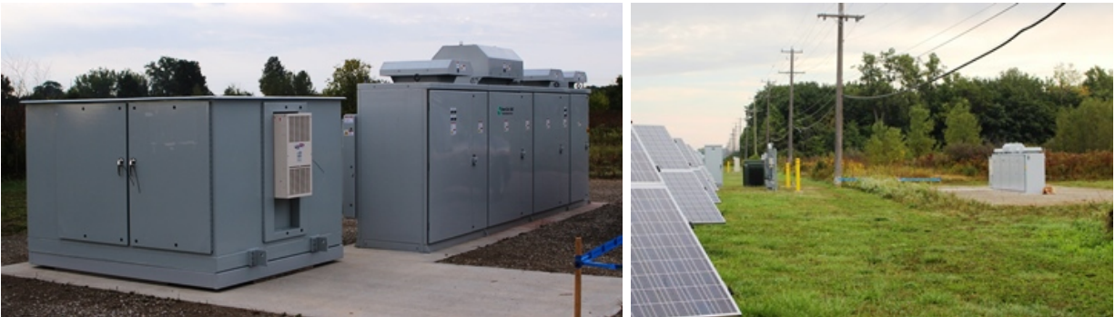
Figure 11: DTE 500 kW system collocated with a 500 kW PV [9].
