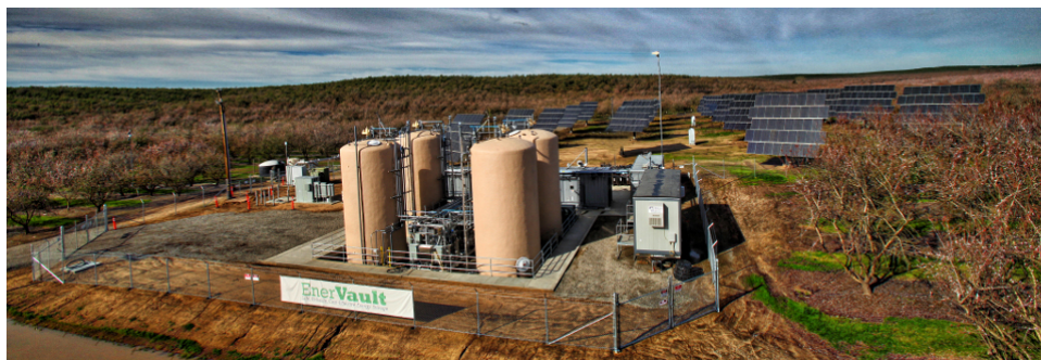
Figure 8: EnerVault Fe-Cr Redox flow battery, Turlock, [7].
