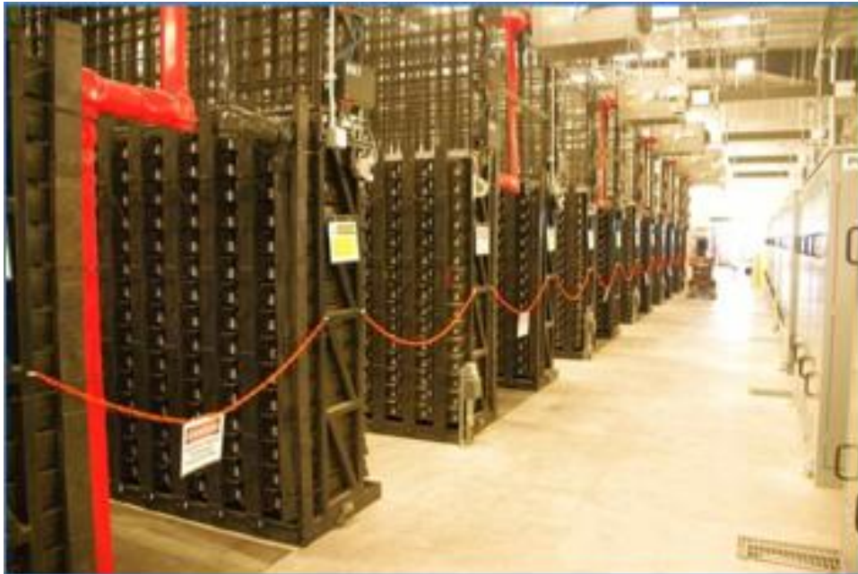
Figure 6: PowerCell Modules at the Duke NoTrees Wind Storage Project [5].
