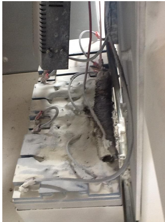
Figure 12 Observed Source of Fire
