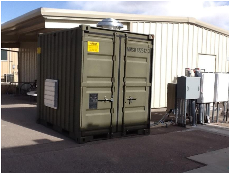
Figure 1 Raytheon/KTech energy storage system delivered to Sandia
