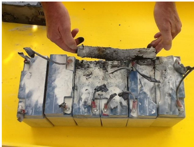
Figure 14 Resistor Fire Fell on Batteries
