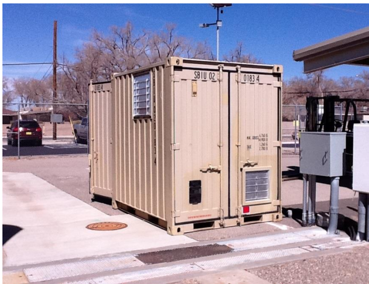
Figure 1 Princeton Power energy storage system delivered to Sandia
