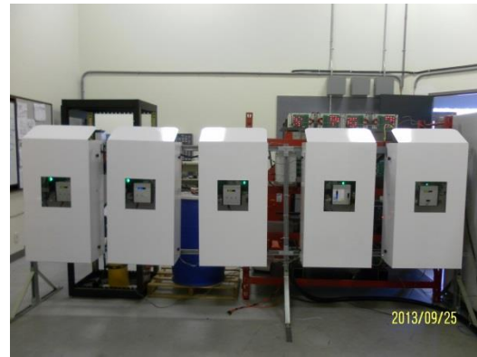
Figure 3 Dc -Dc converters
