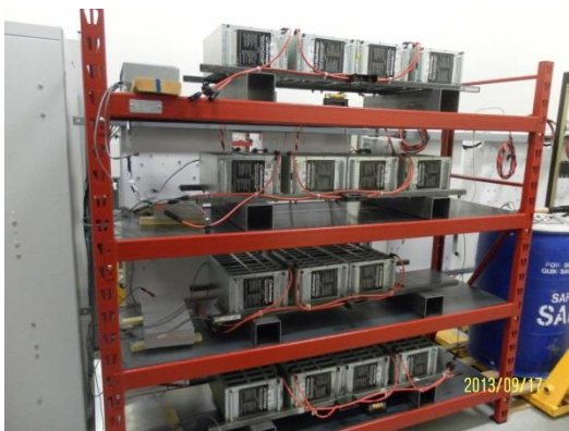
Figure 2: Four Battery packs, with BMS interfaces
