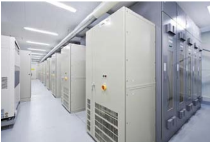
Fig. 2. Photo of Li-ion battery system in the energy storage building.
