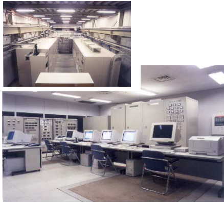
Fig.6. AC/DC converter and control system.
