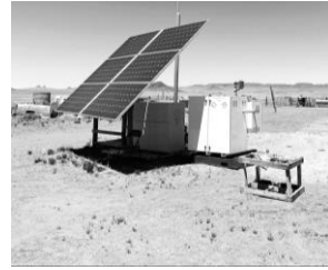
Remote Energy Storage PCS
