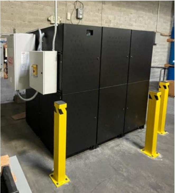
A 20kW/80kWh system In Ogden, Utah
