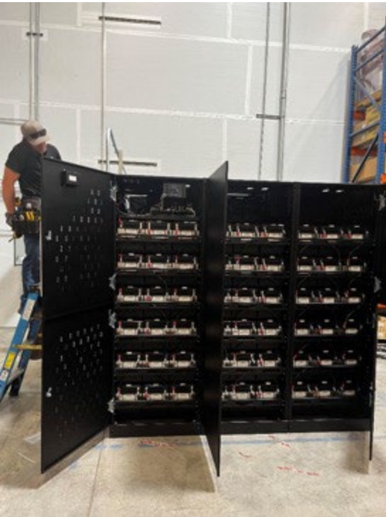
A 20kW/80kWh system In Salt Lake City, Utah
