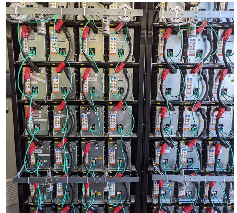
FREQCON BATTERIES MODULES RACKED
