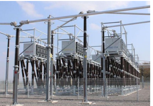
POWER FLOW CONTROL Smart Wires
