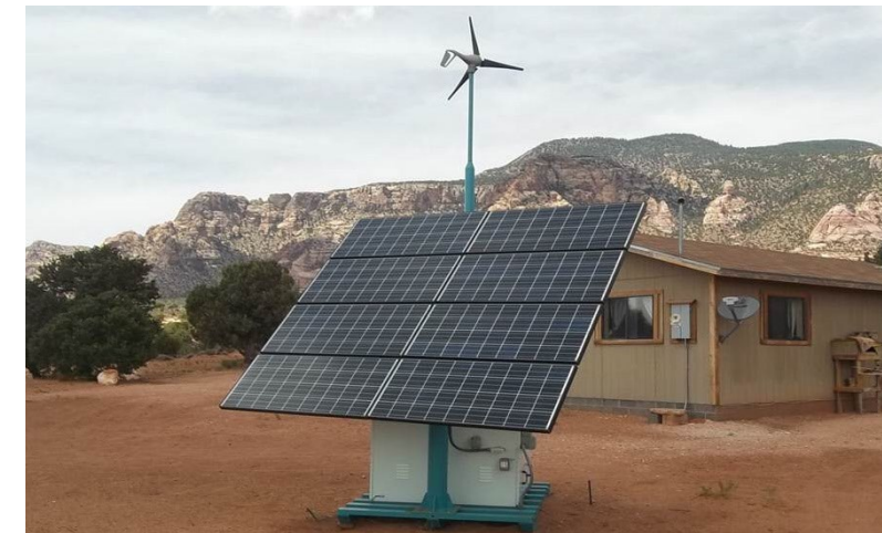
Example Off-Grid Electricity Solution 3
