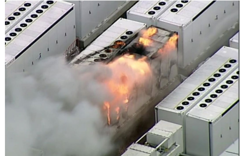
Battery fire: EPRI BESS Failure Event Database*
