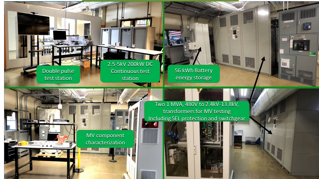
Medium voltage Lab Setup in GRID-C @ ORNL
