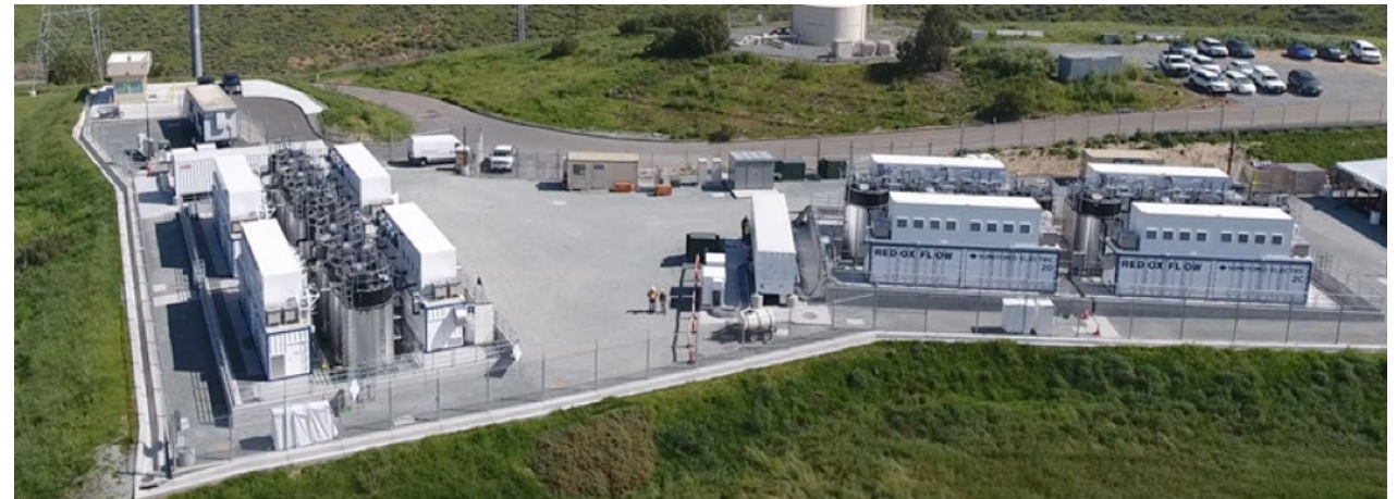
Representative 2MW/8MWhr Vanadium Redox Flow battery system
