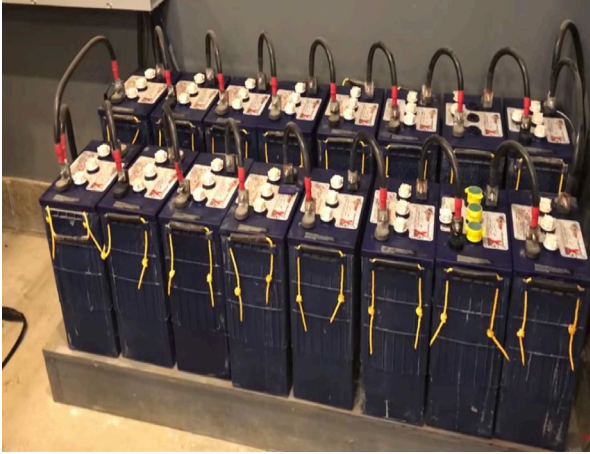
Lead Acid Battery
