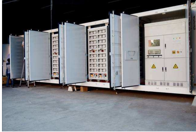
Li-Ion Battery Energy Storage System
