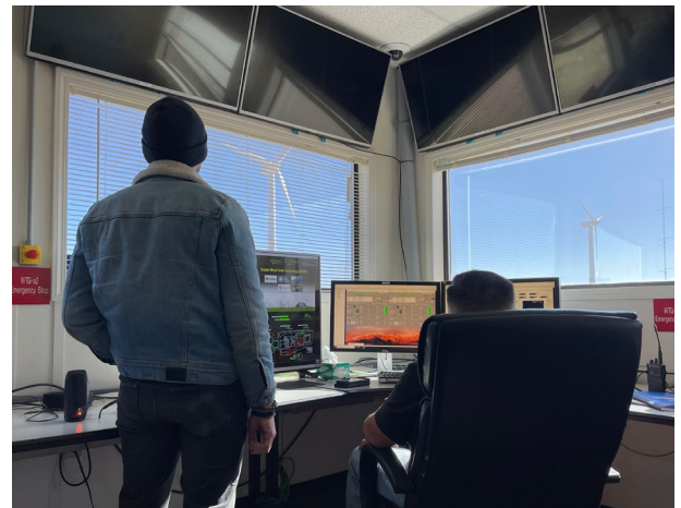
GRID CONTROL — Sandia researchers Rachid Darbali-Zamora and Miguel Jimenez-Aparicio tested AI controls on a microgrid at Texas Tech University. The test demonstrated the system’s ability to manage energy flows in real time.
