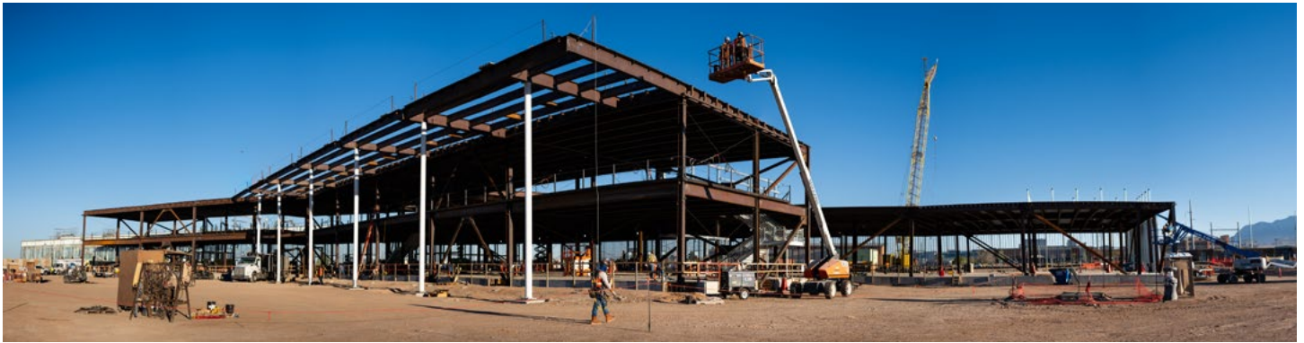
AHEAD OF SCHEDULE — Construction on the 136,000-square-foot Power Sources Capability Building at Sandia is ahead of schedule. A beam ceremony, which signifies completion of the building's steel structure, was held on April 14. Photo by Craig Fritz
