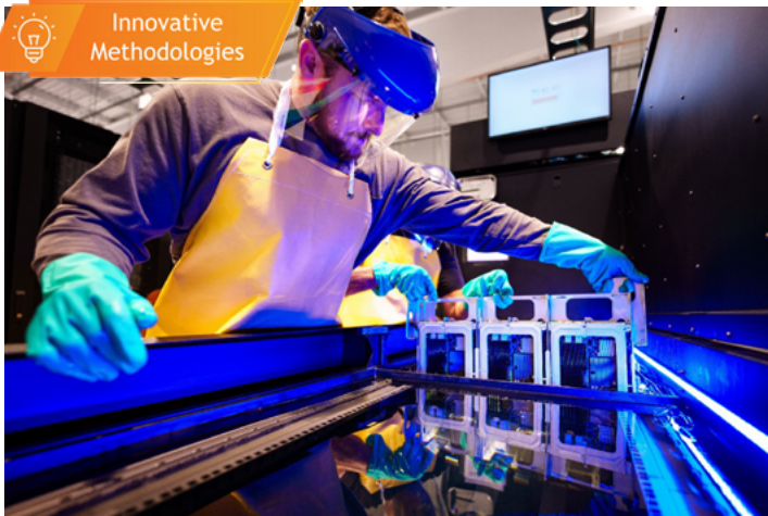
COOLING OFF — David Smith, front, and Dave Martinez, behind, work on a computer server submerged in liquid as part of testing at the High Performance Computing center at Sandia. The immersion system uses a nonconductive liquid coolant that enables 100% of the heat generated to be captured. The reflection of the computer demonstrates the high liquid level. Photo by Craig Fritz
