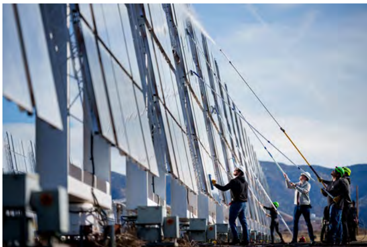
ALL HANDS ON DECK — A group at the National Solar Thermal Test Facility cleans all the heliostats with a power washer, scrubbers and squeegees the morning before a critical test in an attempt to maximize the sun's heat on Dec. 4.
