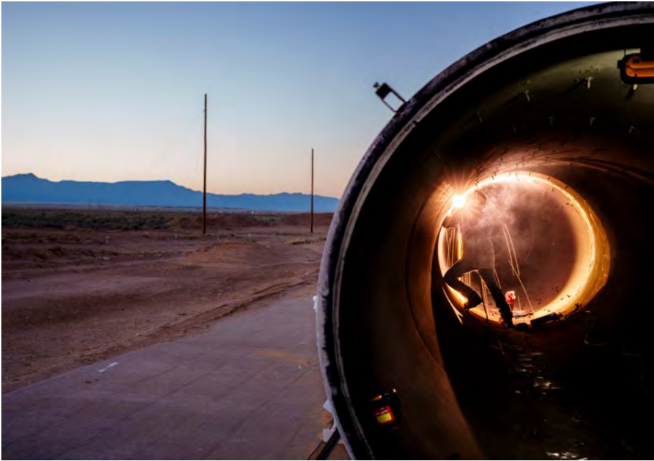
RISE AND GRIND — In preparation for a series of 300-foot blast tube proficiency tests, technologist T.J. King welds a portion of the tube on a September morning.
