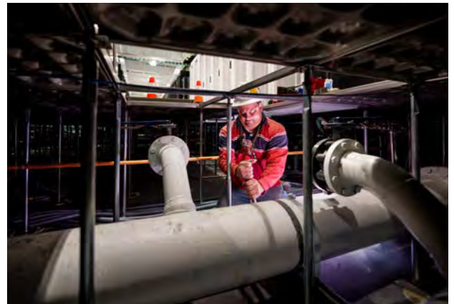
HIGH PERFORMANCE — Gary Roberts, a plumbing contractor, works on the cooling system in Sandia's high-performance computing building on Oct. 9. Photo by Craig Fritz
