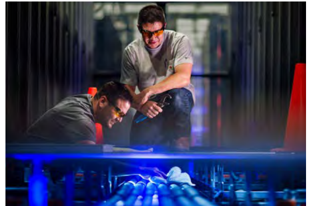
A COOL SYSTEM — Manuel Torres, left and Tony Tafoya check the liquid cooling system in Sandia's high-performance computing building on Oct. 5. As a result of work done on the facility and others, Sandia has been recognized as DOE 50001 Ready site for energy management practices. Photo by Craig Fritz
