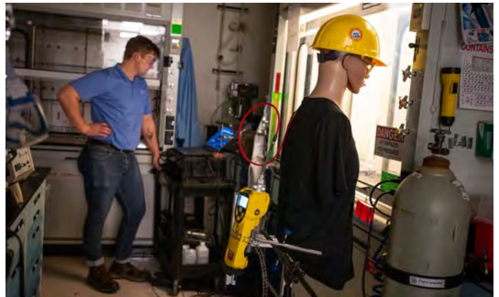
TEST AND ASSESS — Contractor Walker Smith tests fume hoods after performing energy-efficient upgrades as part of the Smart Labs pilot program.
