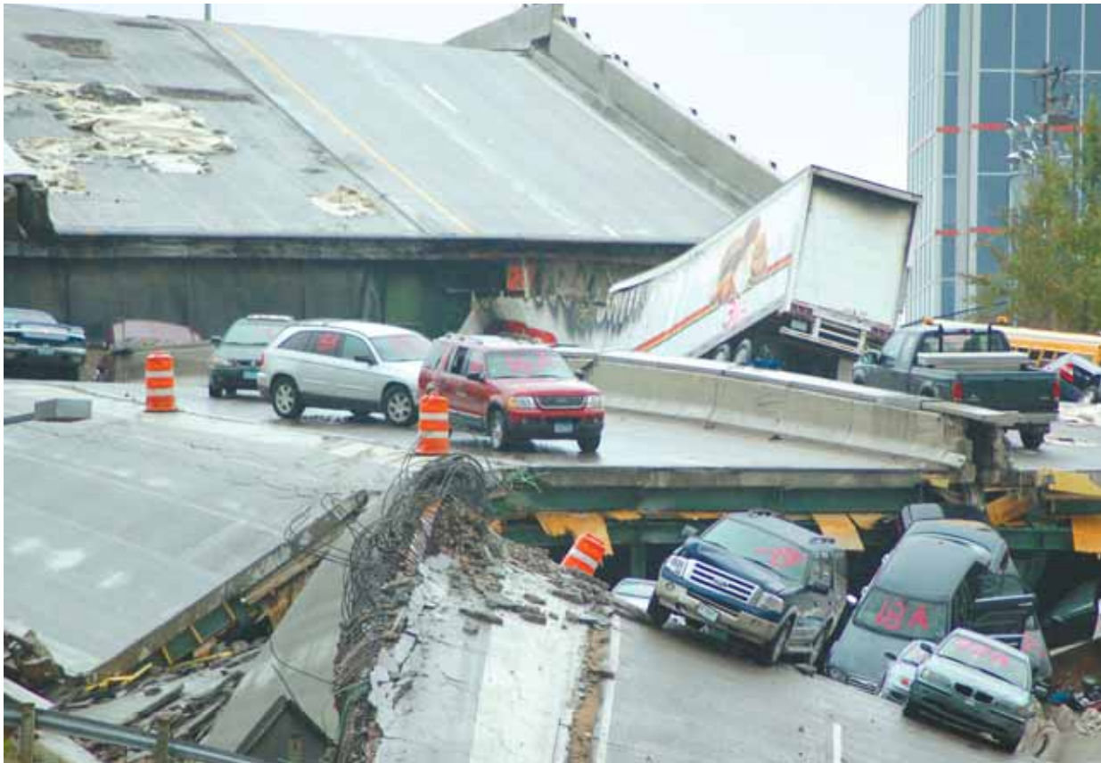
CARS REST on the collapsed portion of the I-35W Mississippi River bridge in Minneapolis, Minn. The photo was taken four days after the Aug. 1, 2007, collapse that claimed 13 lives. (Photo by Kevin Rofidal, US Coast Guard via Wikimedia Commons)
