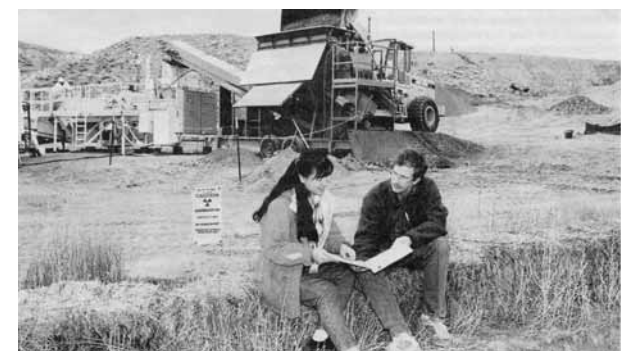
A CLEAN SWEEP — Anh Lai and Fran Nimick look over plans for cleaning up a depleted uranium site in the Tijeras Arroyo. In the background is the Thermo Nuclear rig.
