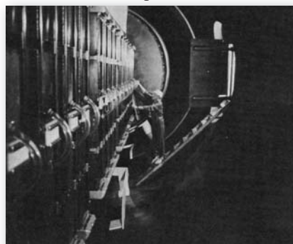
JESSE HARNESS (4233) inspects the new Marx bank of capacitors recently installed in the Hermes II Radiation Simulation Facility.
