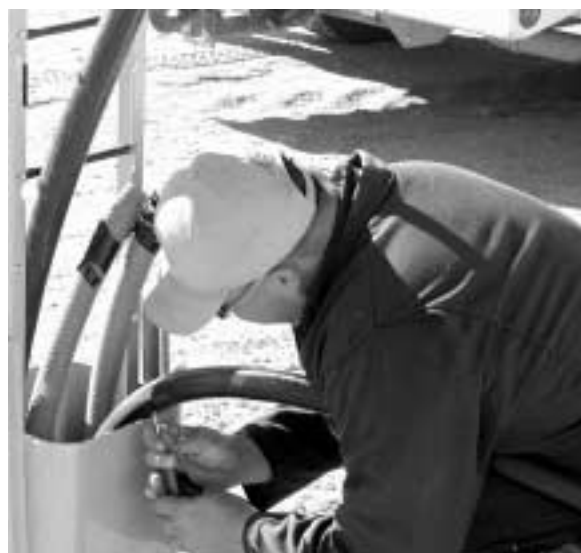
PREPPING A TELEPHONE CABLE for termination in an outside plant pedestal is Carlos Baldonado.
