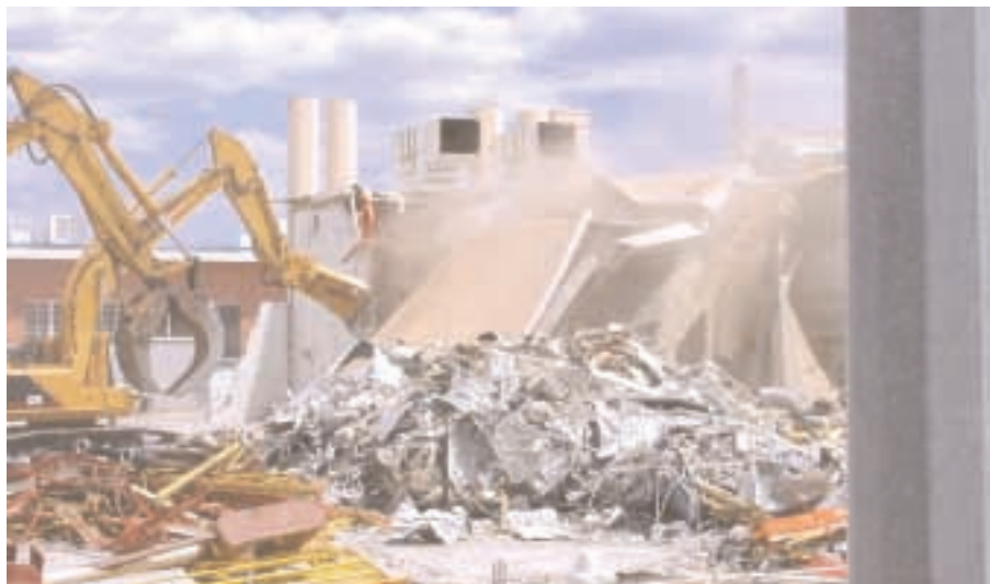
BLDG. 841 meets its doom during the major phase of its demolition. The above-ground part of the demolition began July 8 and took three and a half weeks. However, all the manufacturing services activities that for decades have gone on inside Bldg. 841 — often called "the shops" — have been relocated and are alive and well and ready to serve you in Bldgs. 867, 842, and 840.
