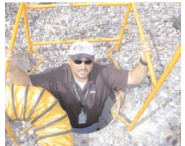
CARLOS BALDONADO exits a manhole that has fiber optic cable. His department, Telecommunications Operations Dept. 9334, was ISO-certified in May.
