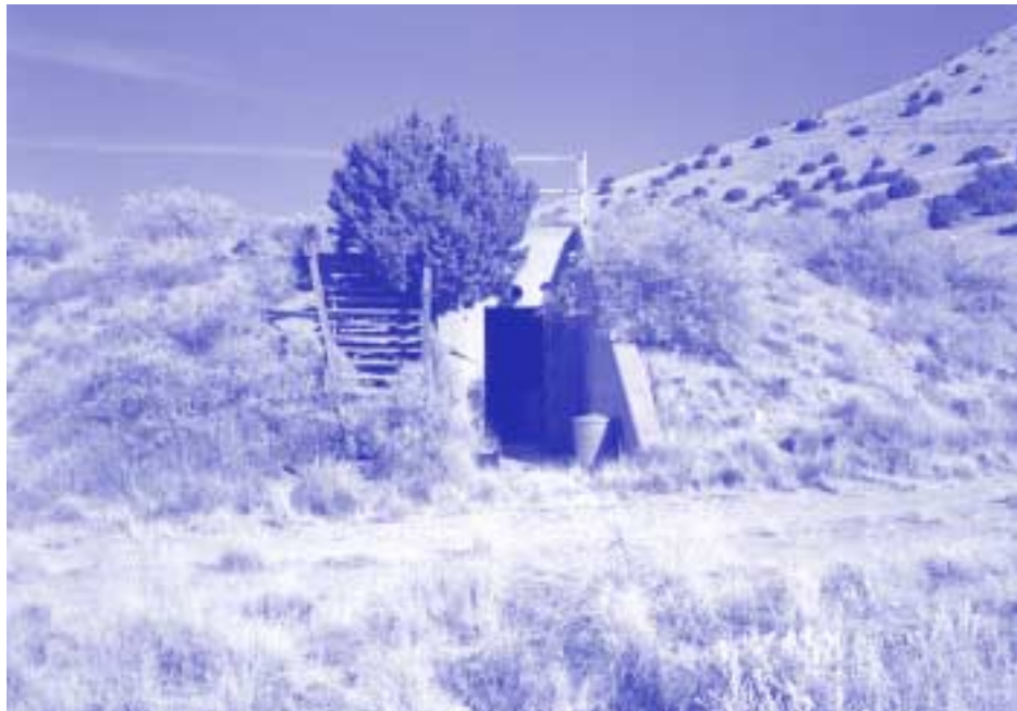
BUILDING 9800B — Located in Sandia's original Coyote Canyon test area, 9800B is contained by berms on three sides lined with steel plating. Unused for several decades, the test facility went up in 1964 and 1965 as a part of the "Halo" test series. More information on activities at the site would be helpful to Sandia historians documenting the site.
