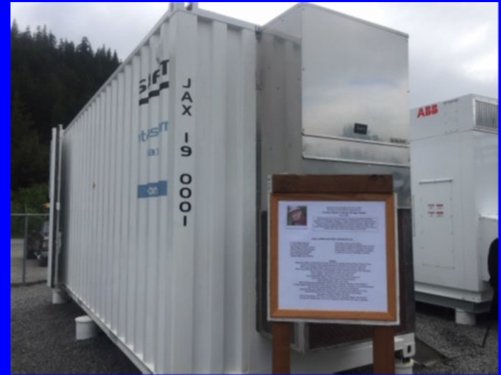
1 MW / 1 hr Li-ion Storage
