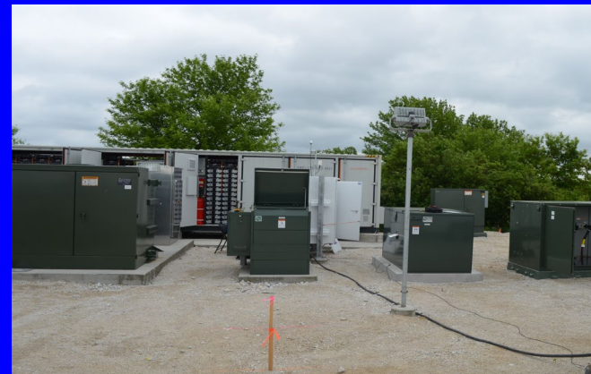
Li-ion batteries by ENEL-X
