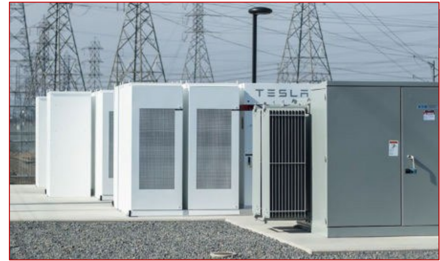
SCE/Tesla 20MW - 80MWh Mira Loma Battery Facility
