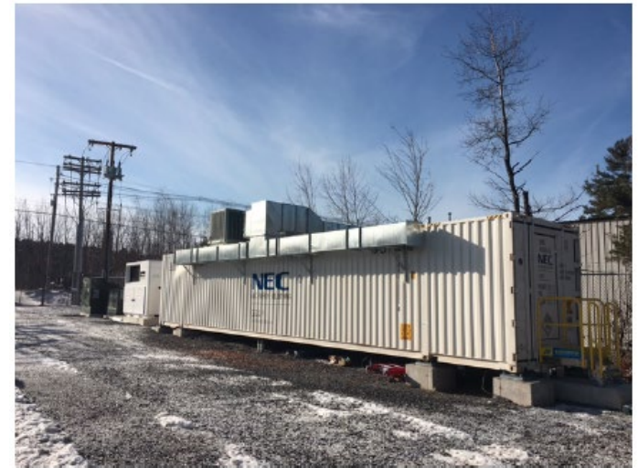
Sterling Municipal Light Department 2 MW, 3.9 MWh system
