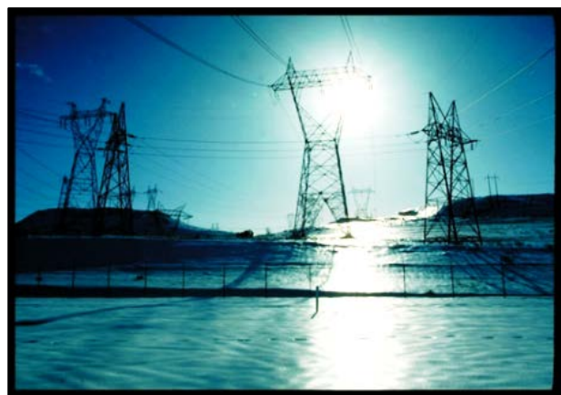
Figure 13: High Voltage Transmission Towers
