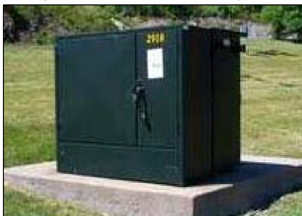
Figure 24: Pad-Mounted Distribution Transformer
