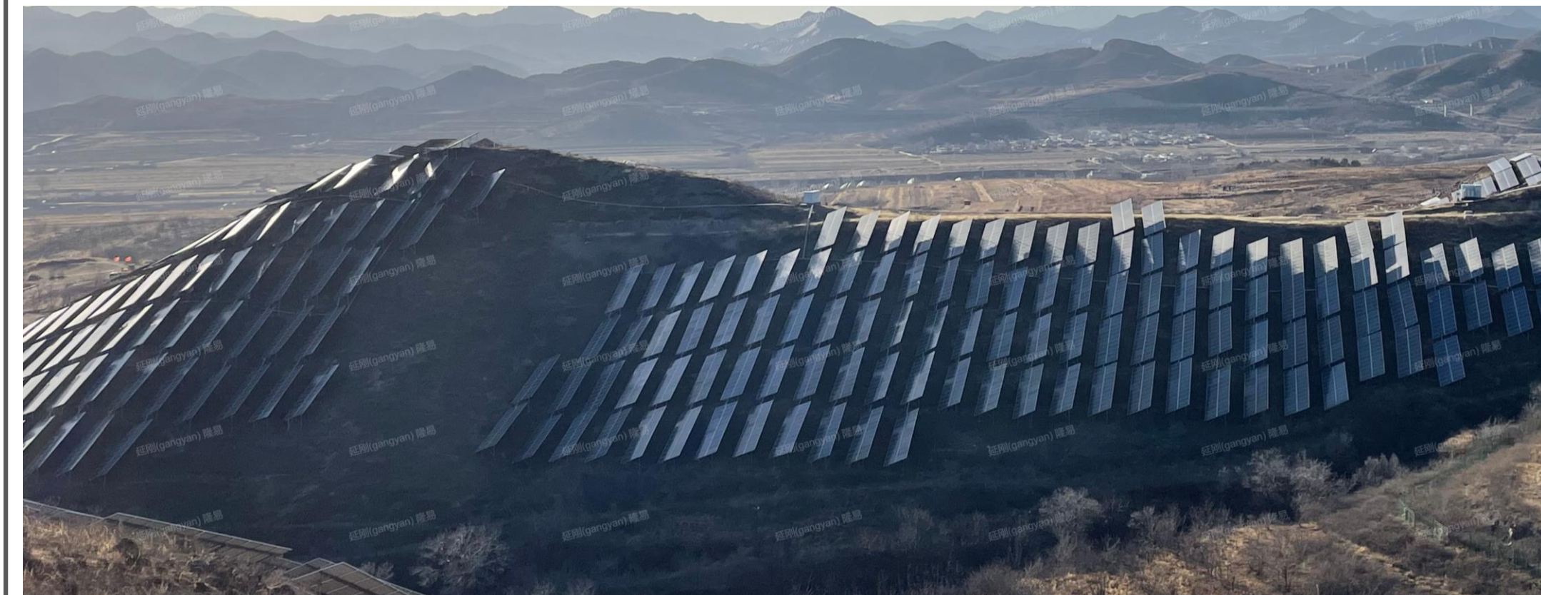
Fig. 1. A terrain PV system in northeast China
