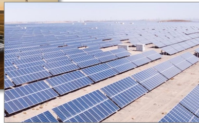
Kingfield Solar Portfolio (Excelsior Energy, Minnesota , US)
