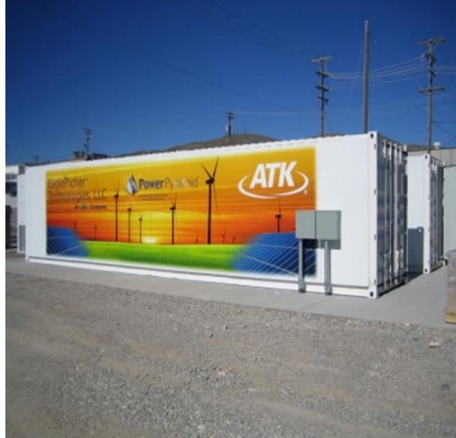
Figure 4.2. ATK BESS System
