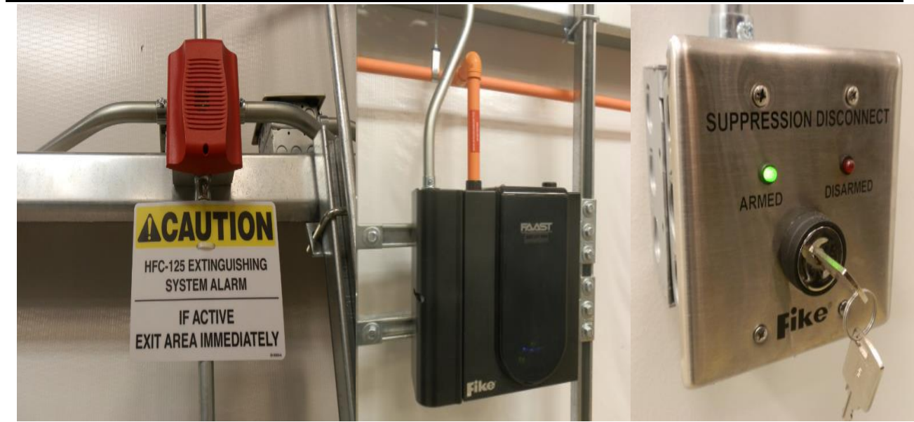
FE-25 Pre-Action Alarm
