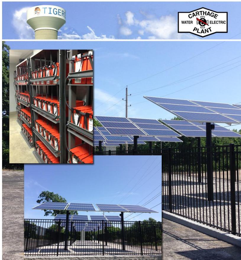
Figure 4.3. CWEP RESS Installation
