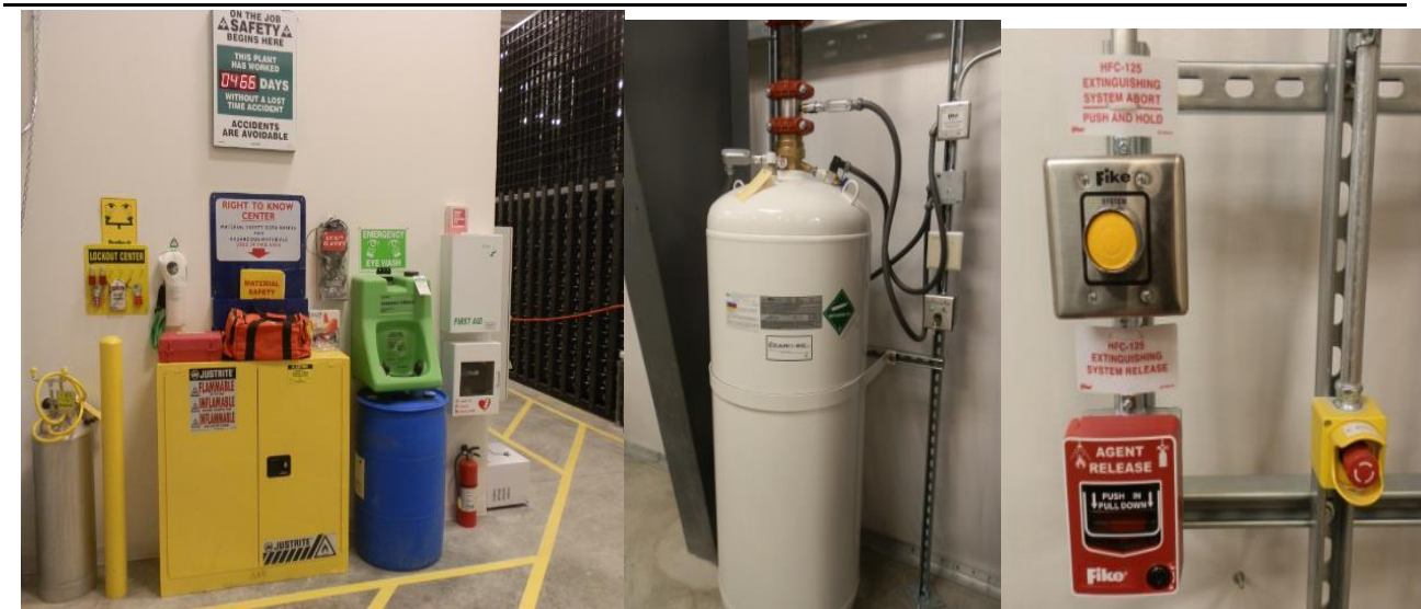
BESS Safety Area
