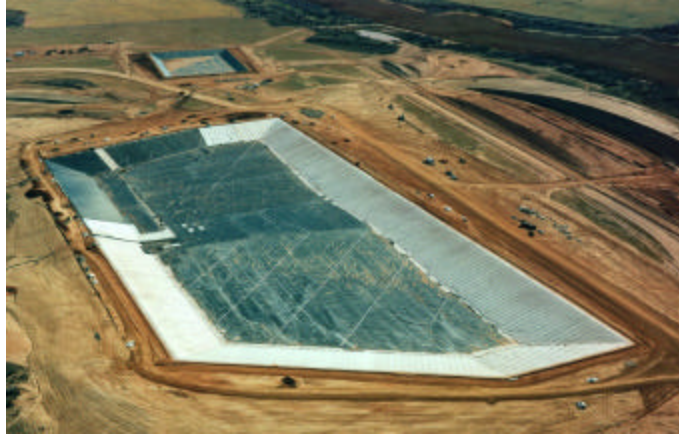
Figure 3. Aerial view of the double composite-liner system at the base of the repository.
