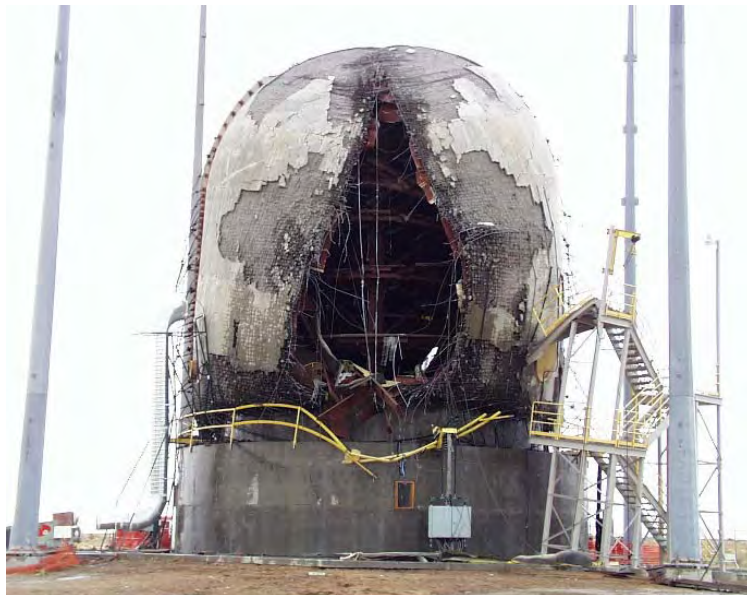
Figure 63 PCCV Model after the Structural Failure Mode Test
