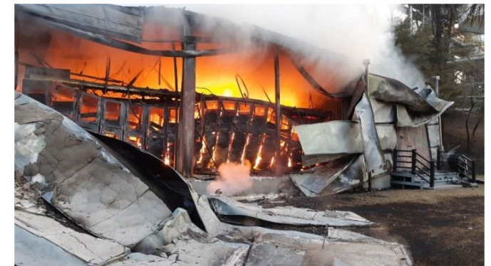
A fire engulfs an energy storage system at a cement plant in Jecheon, North Chungcheong Province, Monday. / Courtesy of North Chungcheong Province Fire Service Headquarters
