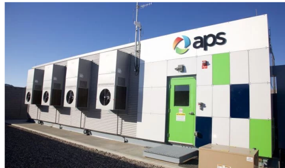
Earlier this year APS announced plans to build 850 megawatts of battery storage by 2025.
