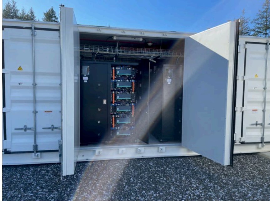
FIGURE 4 Decatur Island Energy Storage System
