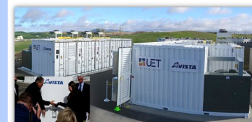
Avista Turner BESS
