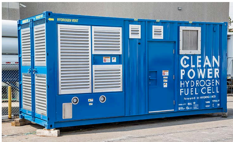
Figure 10. Fuel cell stationary power plant
