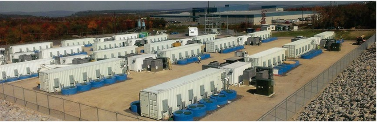
Figure 2. Modern flywheel technology—20 MW flywheel frequency regulation plant (courtesy Beacon Power, LLC)
