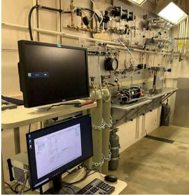
Computer control, data acquisition and piping
