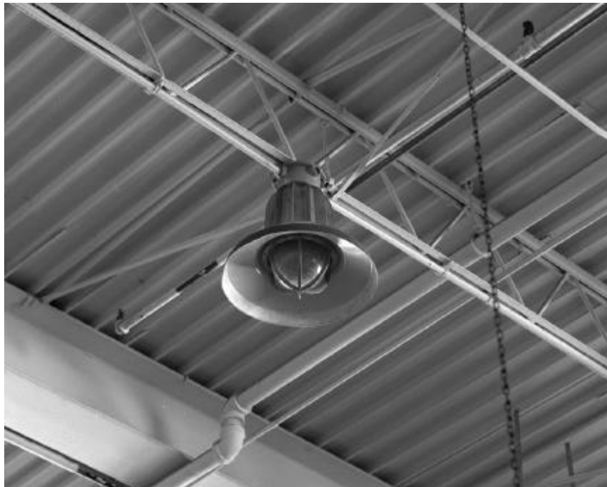
Figure 6. 1997 photo of original light fixture in Building 907 high bay. 47
