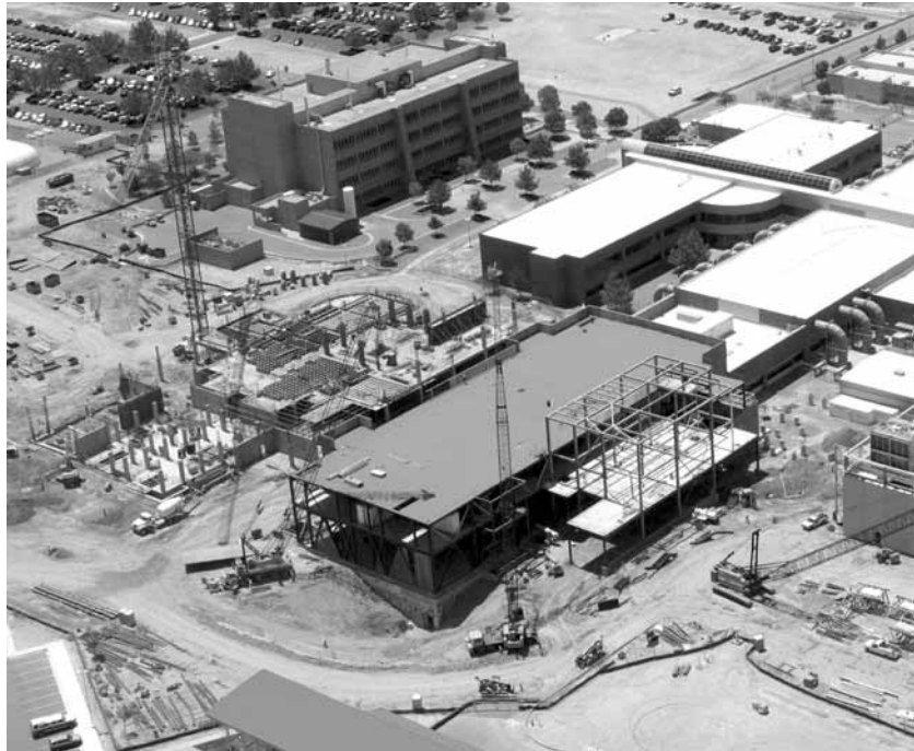
FACILITIES is scrambling to minimize cost, supply impact on Sandia construction projects such as MESA.
