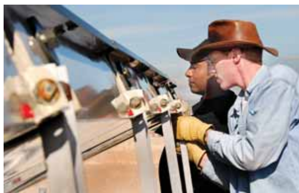
UNM STUDENTS Gehan Kaviratne (left) and Eric Ulrich install the new solar thermal collectors on the roof of UNM's Mechanical Engineering Building.
