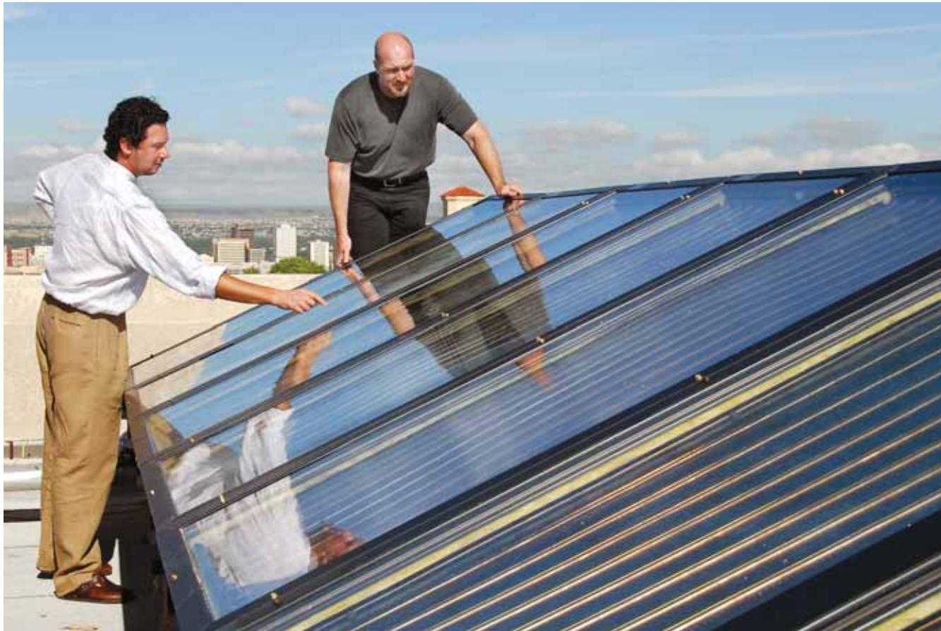
HERE COMES THE SUN — UNM professors Andrea Mammoli (left) and Peter Vorobieff examine solar thermal collectors on the roof of the Mechanical Engineering Building on the campus of the University of New Mexico. Sandia is helping upgrade the solar system to the latest technologies. (Photos by Randy Montoya)
