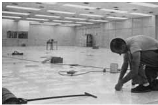
NEARING COMPLETION — The special 705 computer room in Bldg. 880 receives final touches from a construction worker. Removable floor panels allow access to the electrical connections.
