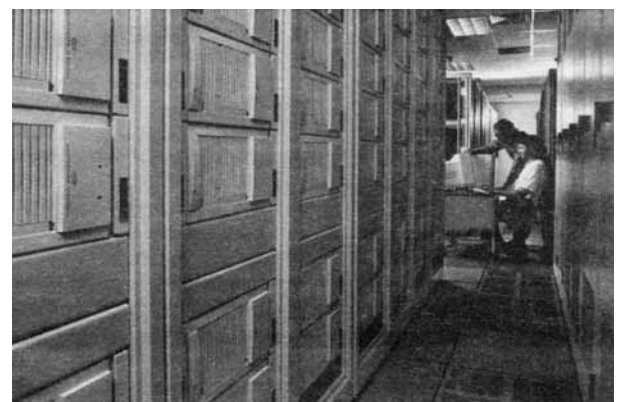
CPLANT PATCH — Rolf Riesen (standing) and Ron Brightwell monitor computations being performed on Sandia's Cplant. (Photo by Randy Montoya)
