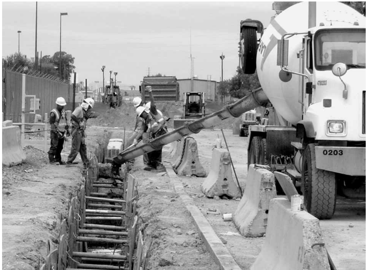
ECIM CONSTRUCTION WORK took 31 months to complete. The underground work involved tearing up streets, sidewalks, landscaped areas, and parking lots and trenching as deep as 16 feet so that duct banks could be installed. (Photo by David Hendrix)
