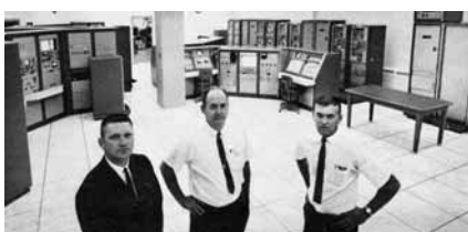
NEW CONTROL CENTER for acoustic and vibration test facilities in Area III. From left are John Otts, test operations supervisor; George Lemmon, facility designer; and Ken Bauhs, responsible for data systems design.
