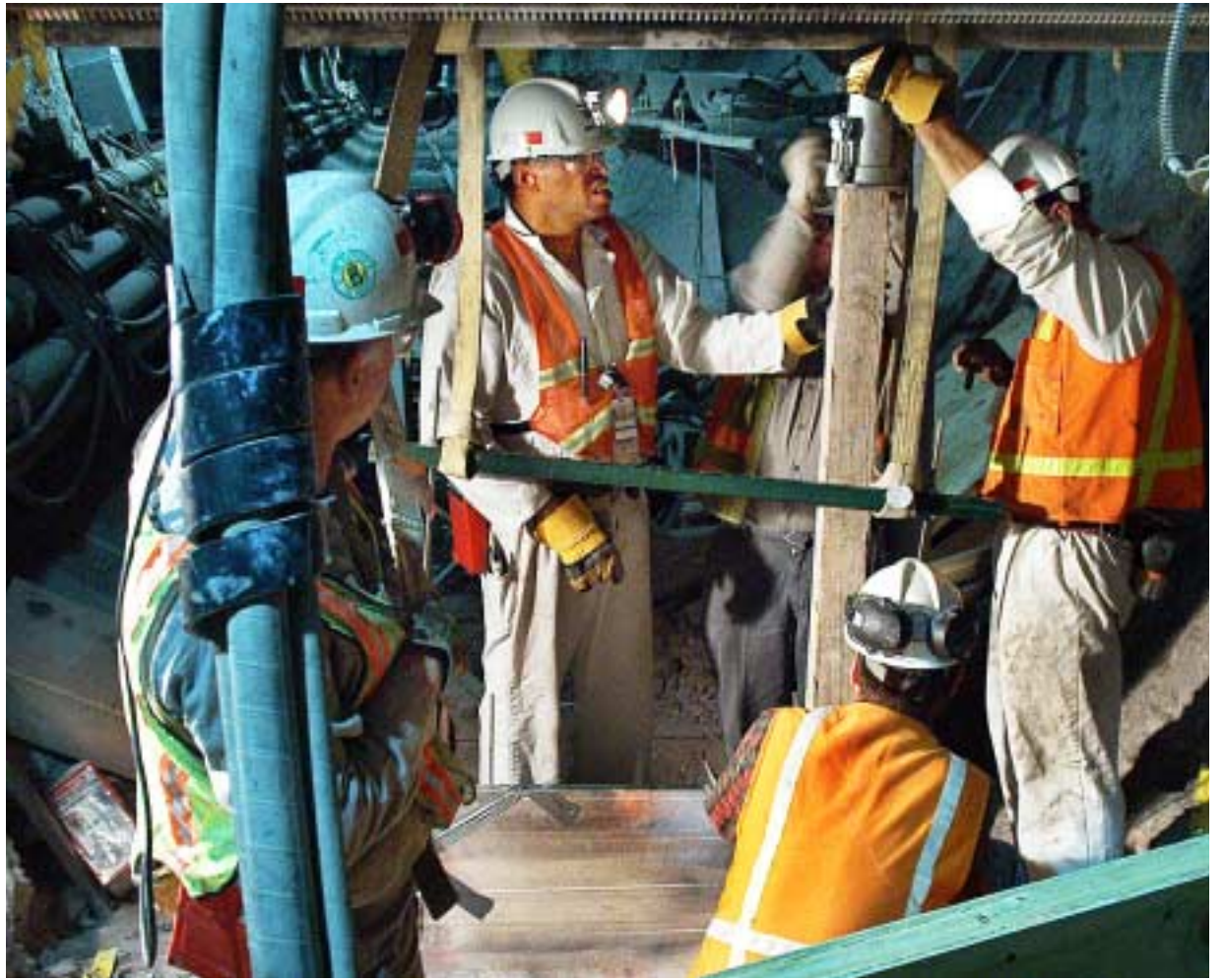
TIGHT QUARTERS — Ron Taylor (6855, center), Dave Bronowski (6117), and a third worker use some gentle persuasion to insert a one-meter-square flat jack into a slot cut in the rock of a Yucca Mountain exploratory drift. The two onlookers in foreground are from the Test Coordination Office, which is run by Los Alamos National Laboratory.
